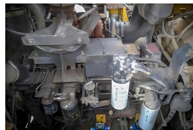
Rear engine fuel system rear of Komatsu and installed flow meters
